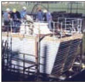
Lakeside's first cooling tower built under license.
