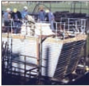
Lakeside's first cooling tower built under license.
